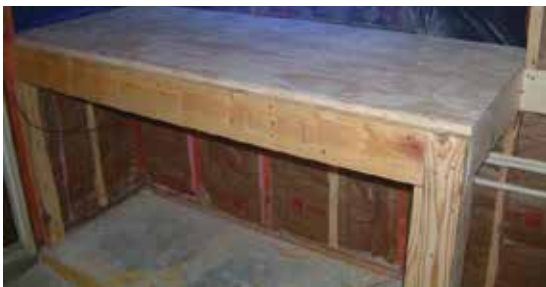
This stand made by a general contractor for a very large and tall aquarium resulted in a failure from the stand warping. It "looks" strong but was inadequate.
